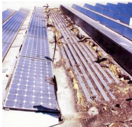
Figure 1.1: Fire hazard in 383 kW PV arrays in Bakersfield, California in 2009
