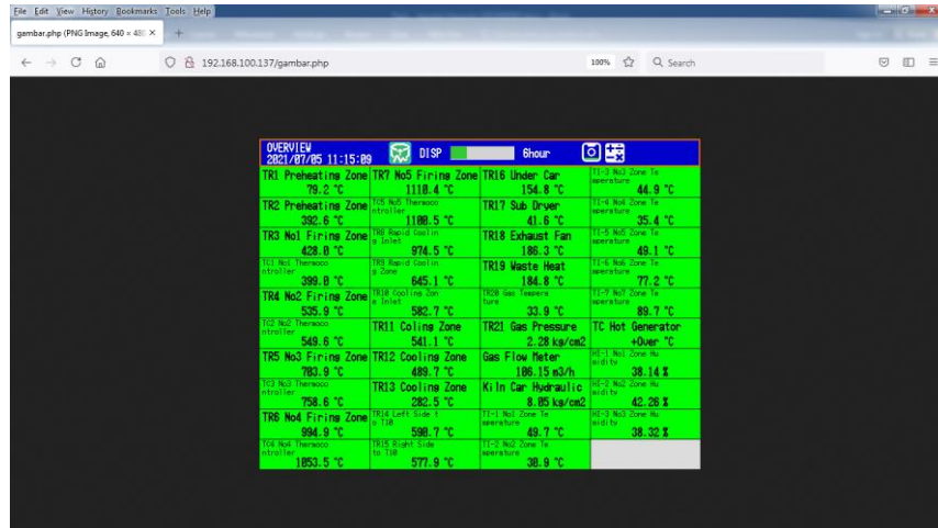
Fig 7. Typical Display of Kiln Machines
